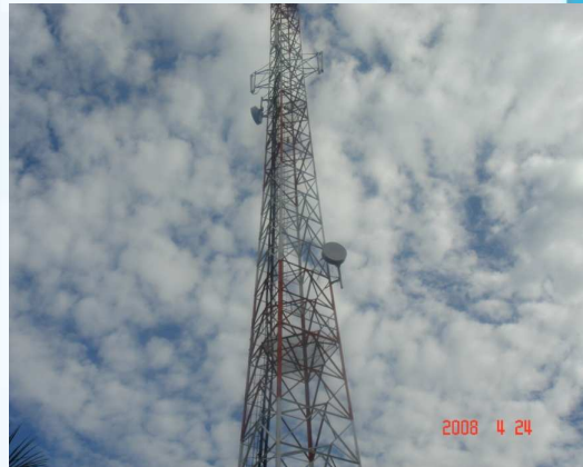
MTN mast at Tororo town, Tororo district
